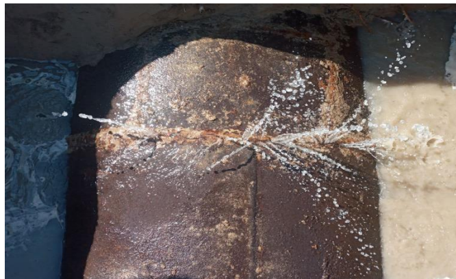
Figure 3. Water hammer on the pressure pipeline; emergency shutdown of the pump and rupture of the pressure pipeline
