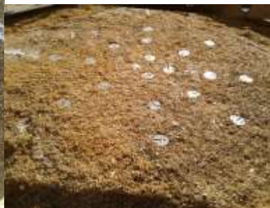
Figure 8. An overview of the springs used as VAEs after installation.
