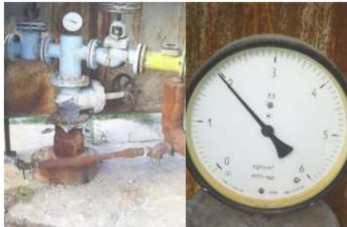
Fig. 4 - View of the geothermal well of the sanatorium "Altyaryk" and pressure readings in the well.
