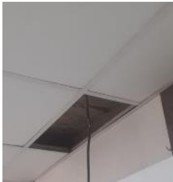
Figure 11: Lack of insulation materials on the roofs
