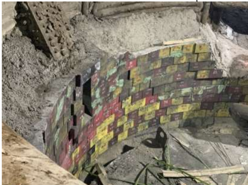
2 – picture. The process of plastering the base lining of an electric arc furnace
